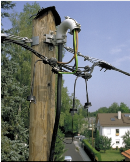
Transition: insulated overhead lines to cables
